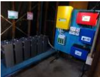
Stand Alone Battery Storage
