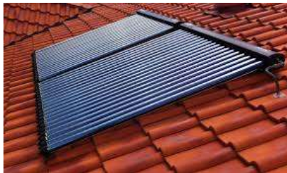
Solar Hot Water
